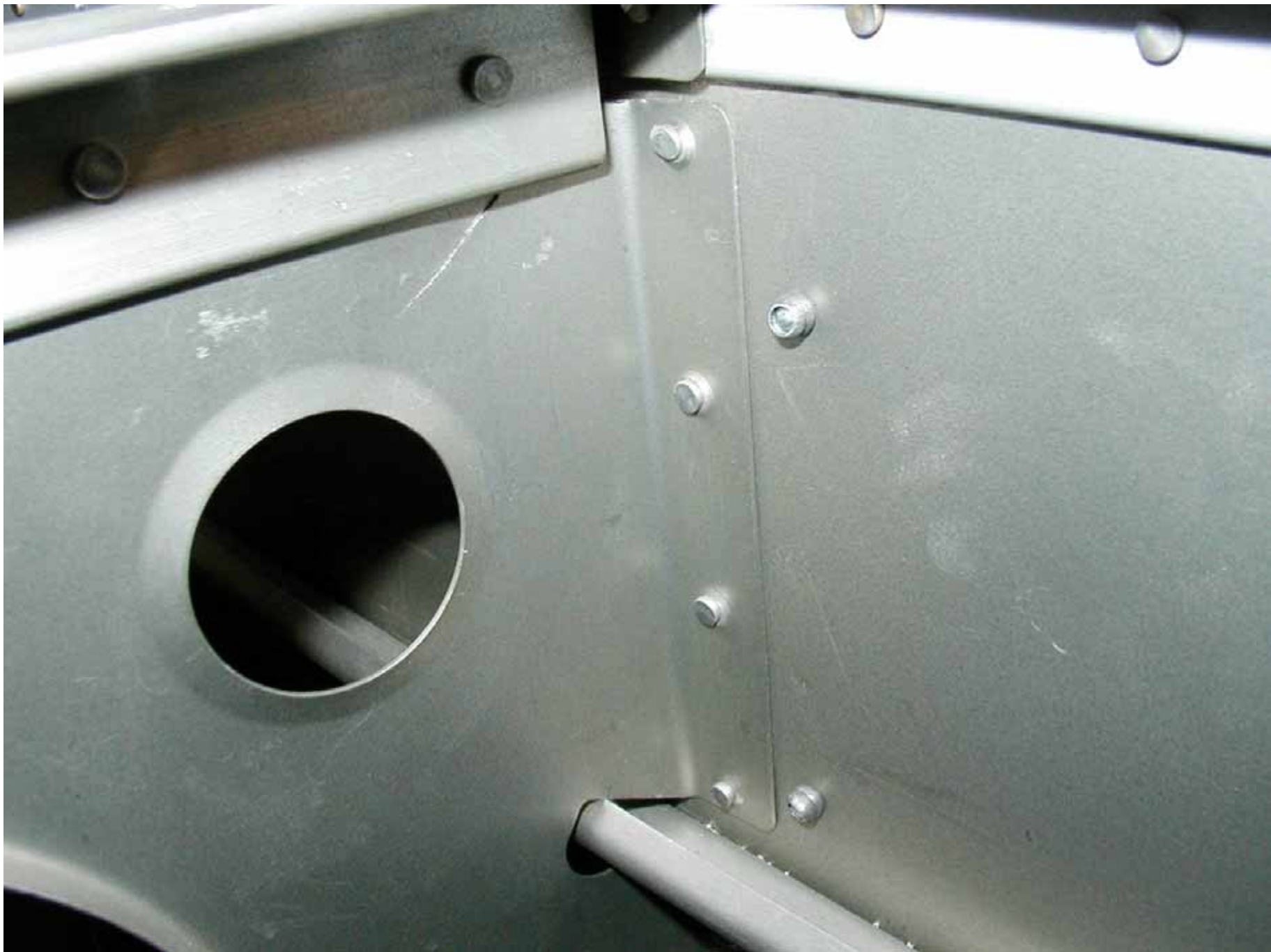
Crack in the upper left corner of F-1010 bulkhead....as seen from the front side looking aft.
